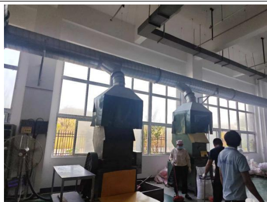
破碎粉尘废气集气罩
